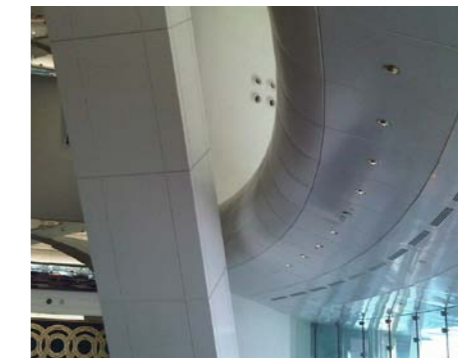
CEILING AND INTERIORS
