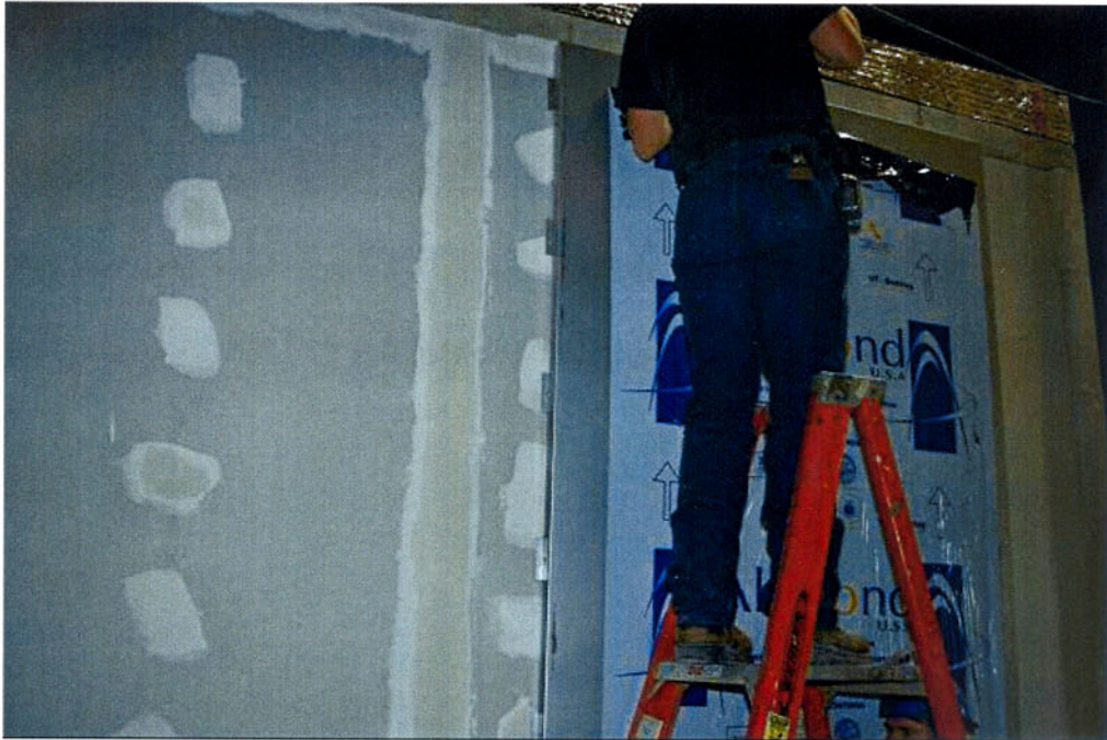
Figure B-5. ACP Panels Being Installed on the Exposed Face of the Wall.
